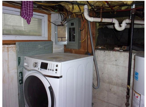
Main House Panel: the area should be clear in front of the panel
