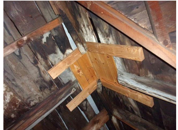
Attic Framing/Sheathing: previous leak and repair
