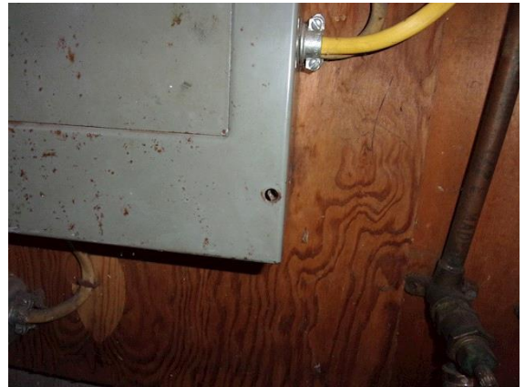
Main House Panel: one missing screw
