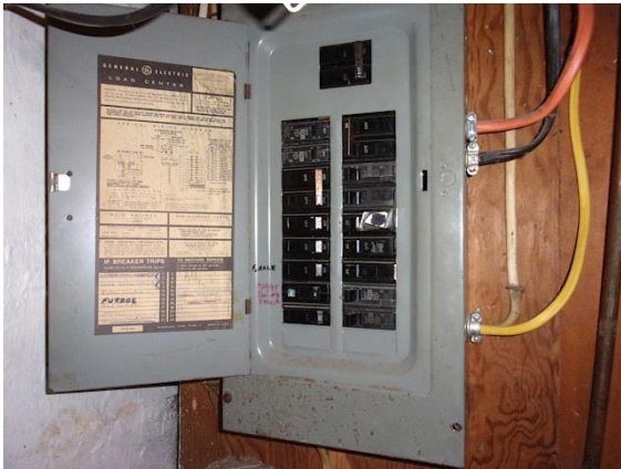
Main House Panel:
